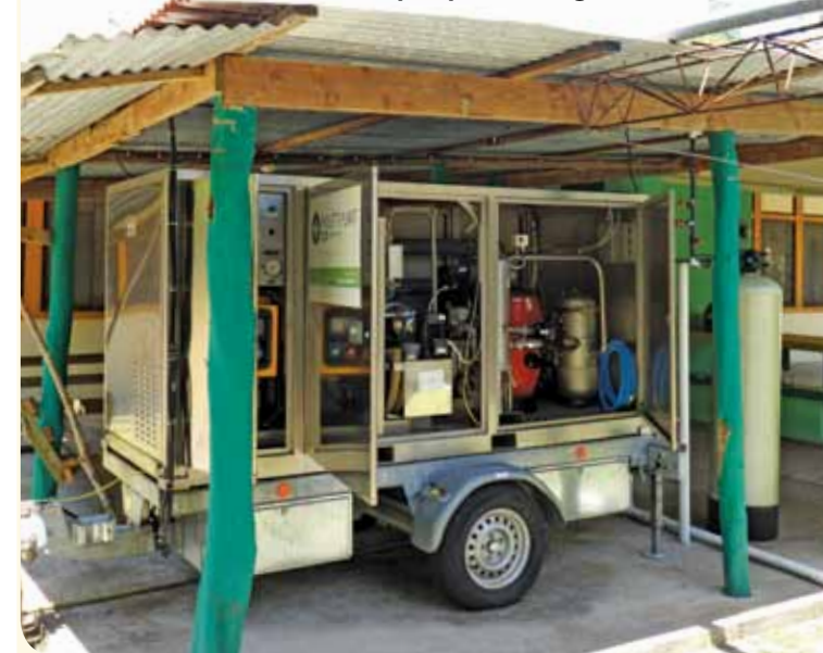
■ Desalination unit that yields the best quality water to people on Angaur Island.
